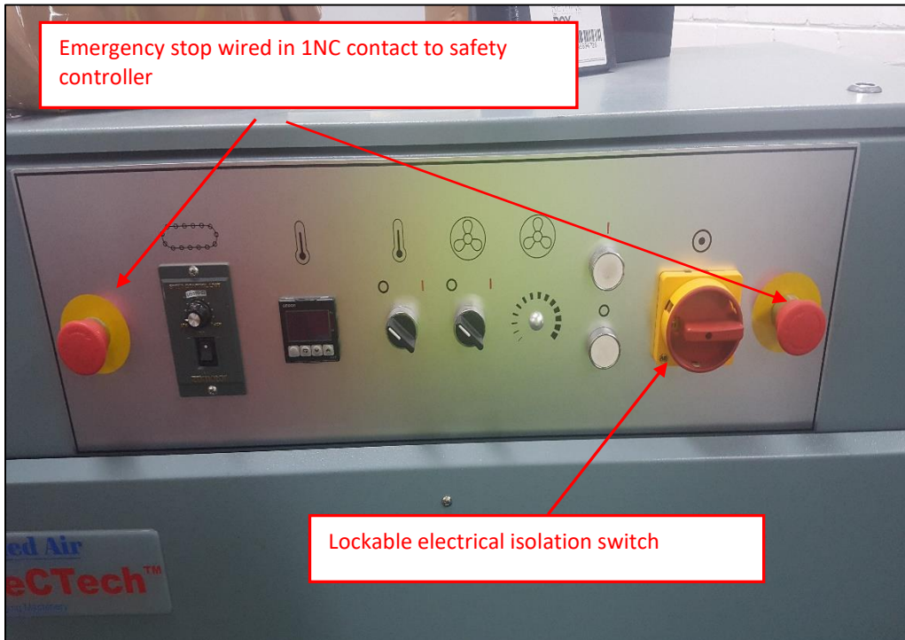
Photo 19: Shrink Tunnel Machine: Operator control panel with Emergency stop
