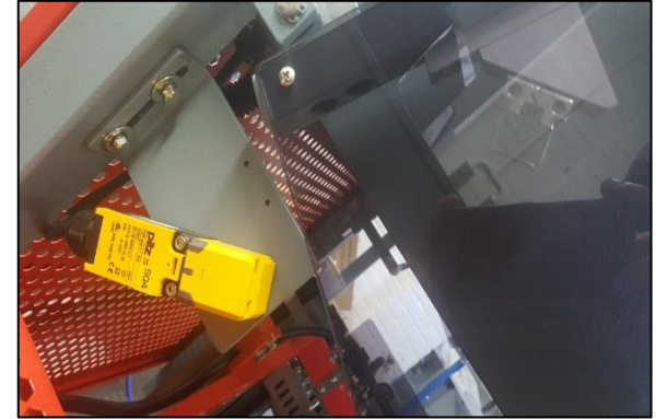
Photo 9: Wrapper SLCT-FA16004: Pilz Psen me4.1/4as safety switch on interlocked guard
