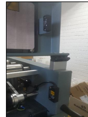
Photo 6: Wrapper SLCT-FA16004: Omron D40A-1C2 guard switch on perforator guard
